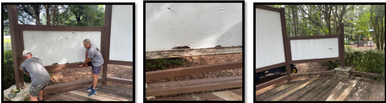
Replace rotting boards.
