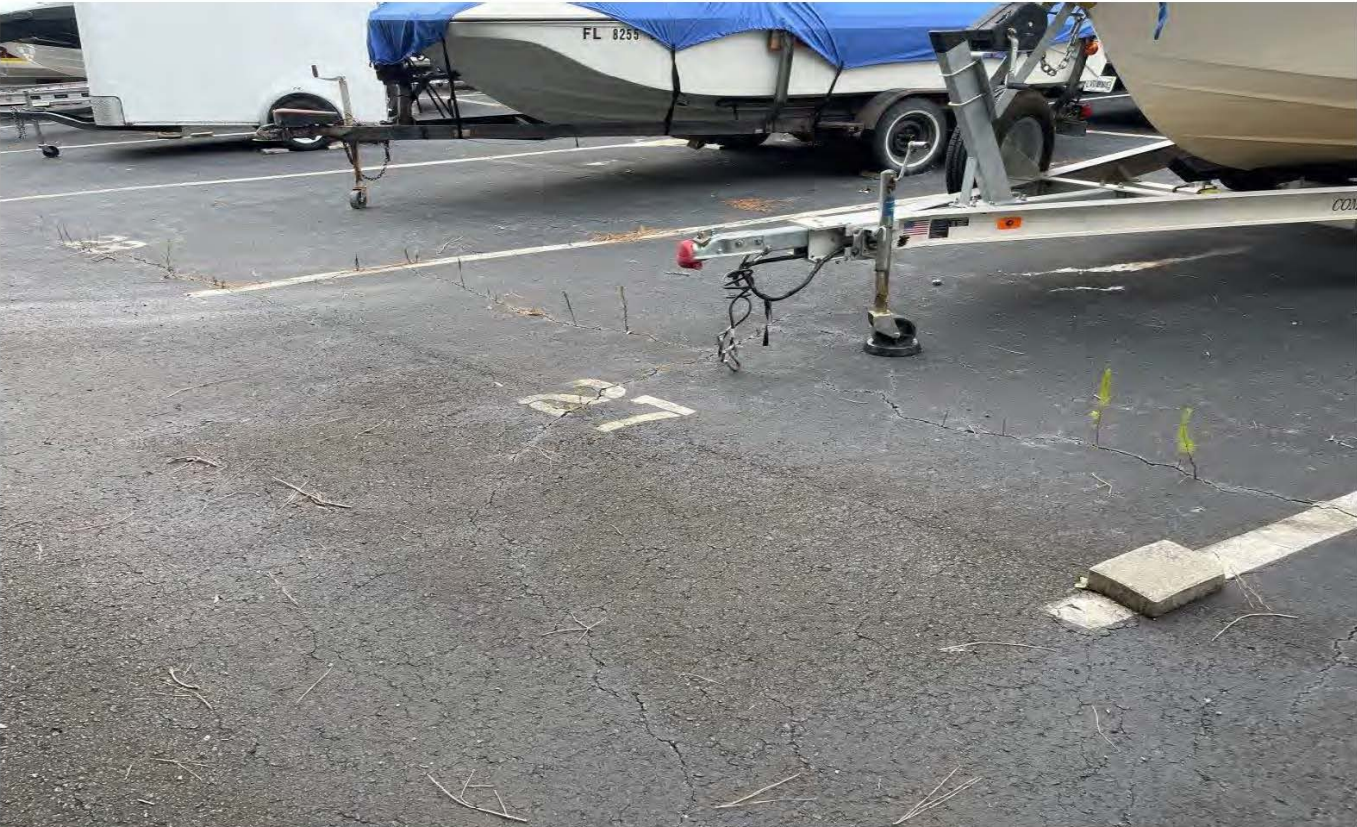
Recreational Boat and RV Parking Bay – Pavement Cracking (06-26-23)
