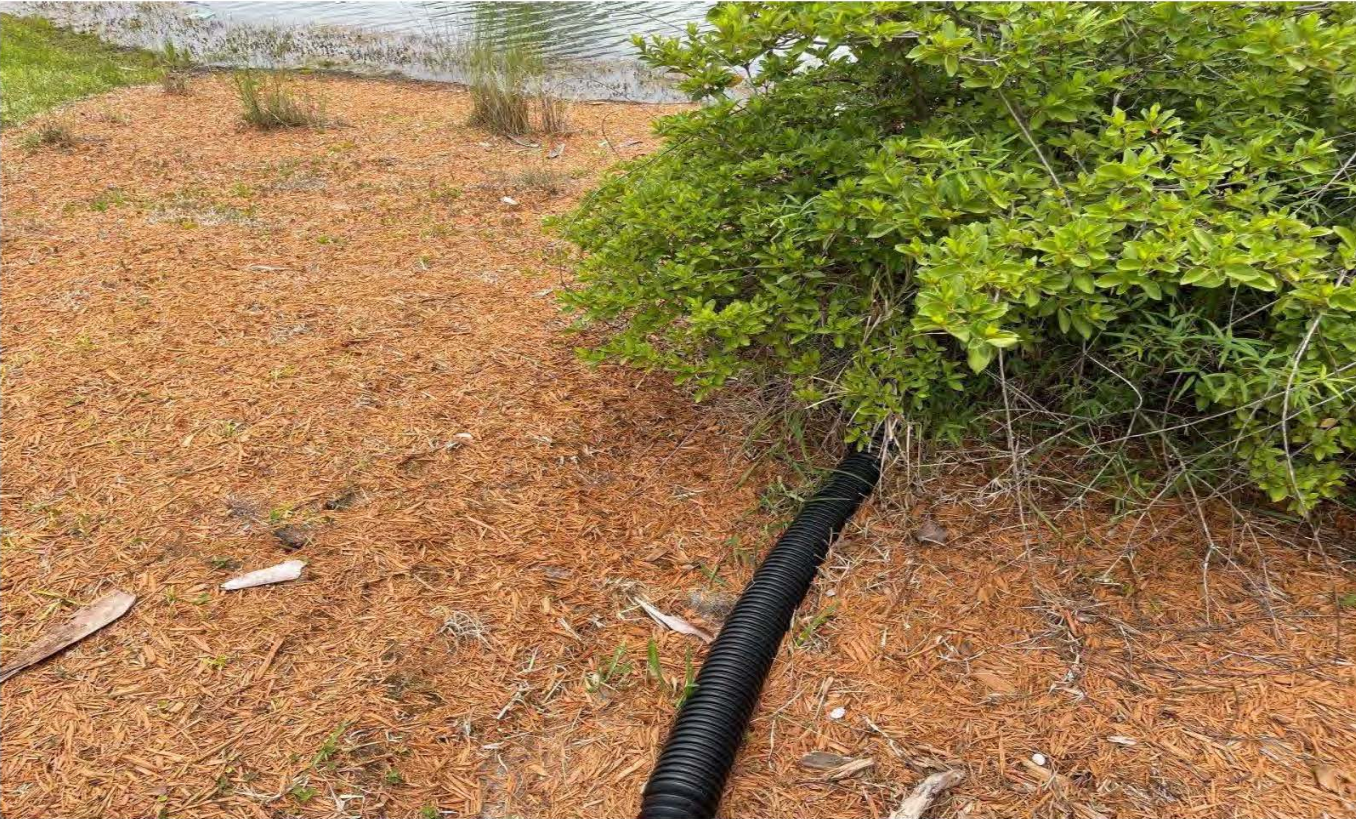
Amenity Center – West Side of Pool Deck (Monitoring Minor Erosion Prevention System) (06-26-23)
