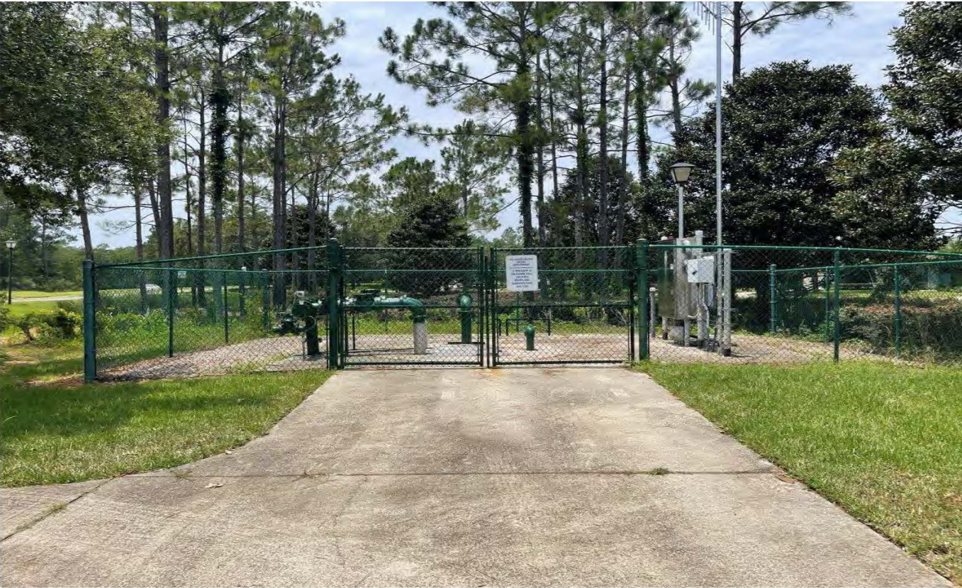
Lift Station on Steamboat Landing Drive (06-26-23)
