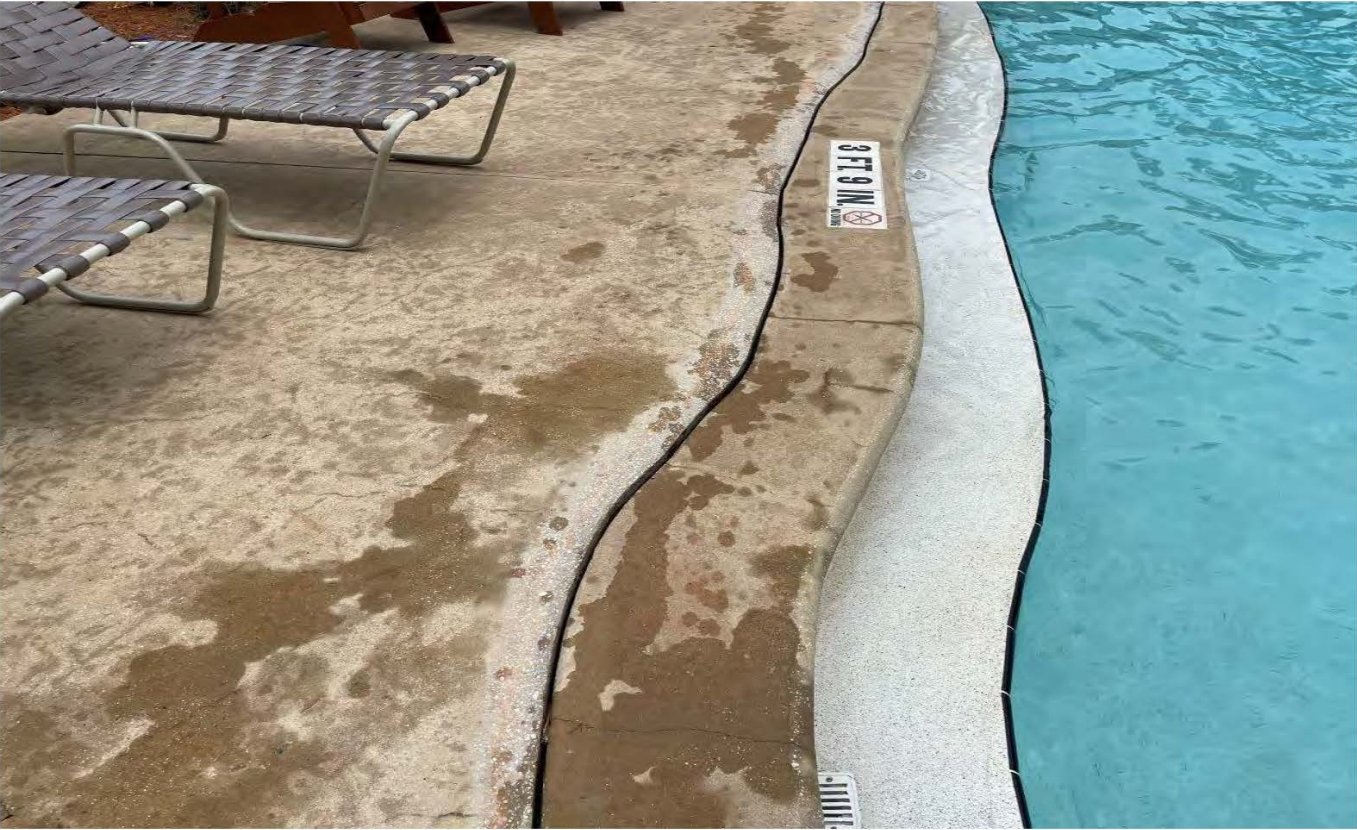
Amenity Center – Pool Deck and Cracking Separation (Monitored by CDD) (06-26-23)
