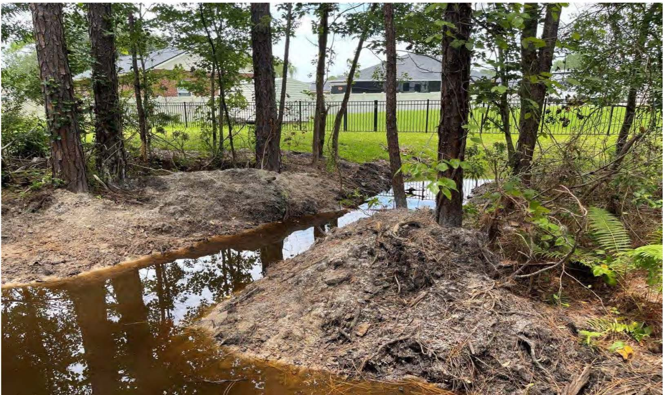
Recently Cleared Drainage Swale – Adjacent to Heritage Landing and Ashley Oaks CDD (Towards County Road 13) (06-26-23)
